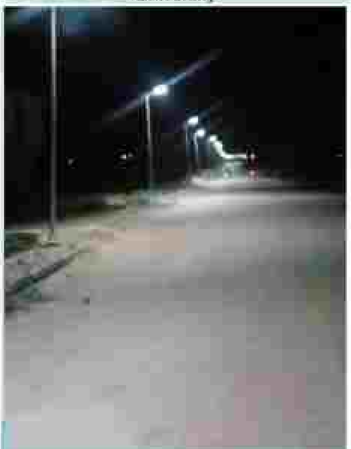
Street lights from Intermediate Staff Quarters to Senior Staff Quarters
