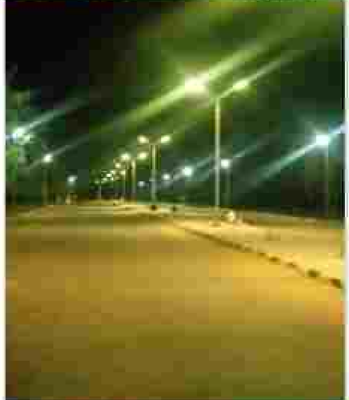
Installed solar street light from the main gate coming in to the University.
